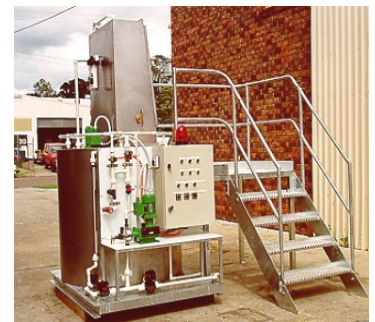
Carbon Dosing System
